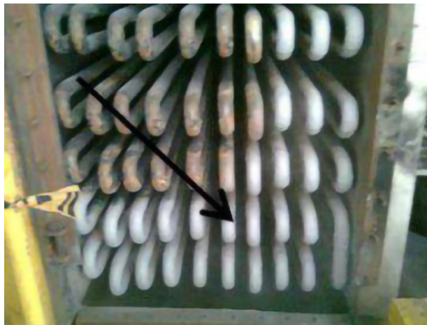
Figure 7. Boiler pipes after one year of operation. Courtesy of Ferresolda
